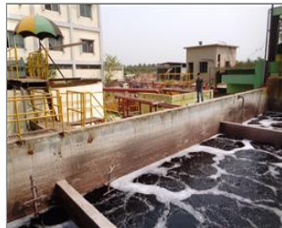
External photo(s) of the production unit(s) ETP area.JPG
