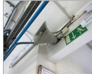
Photo of fire safety equipment PA system.JPG
