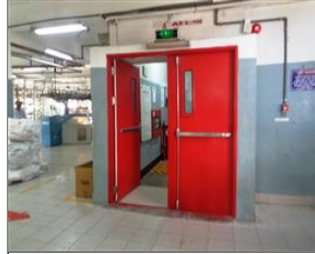
Photo of fire safety equipment Fire proof exit.JPG
