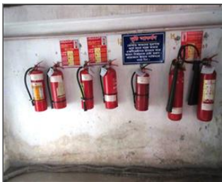
Photo of fire safety equipment ABC and CO2 Type fire extinguisher.JPG
